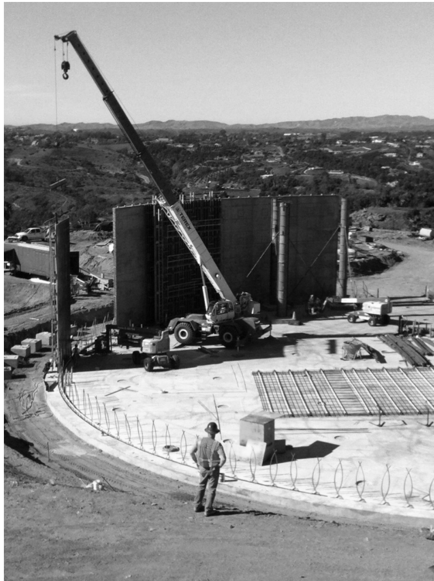
A crane steadies one of the new wall panels at the Pala Mesa Tank
